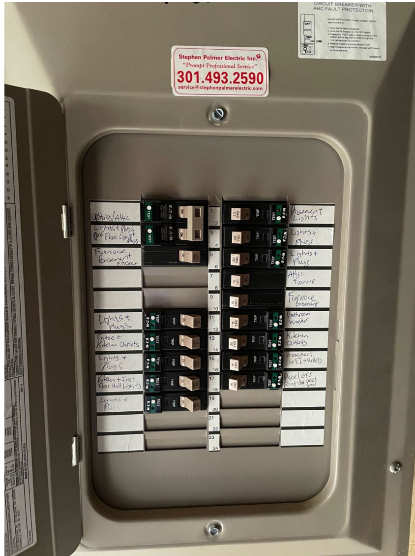
New electrical panel.
