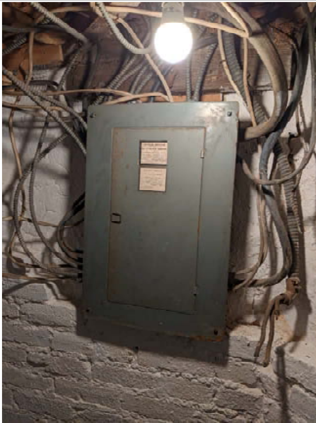
Existing Bryant electrical panel in the basement installed in 1976 (east), which will be replaced. (8/25/2024)
