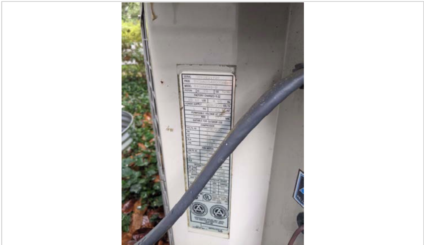
Existing Bryant AC condenser unit (west), which uses R-22 refrigerant. (8/25/2024)
