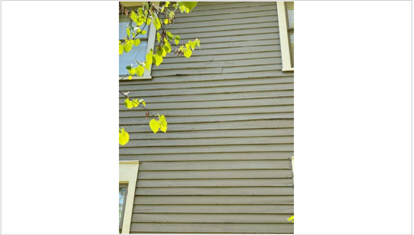
East side - Siding rot
