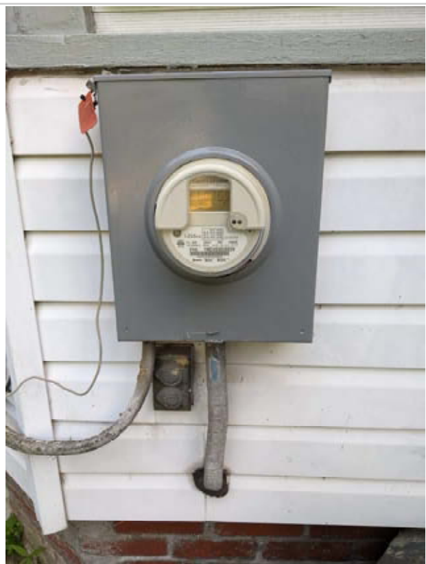
Existing service meter socket and service cable (east), which will be replaced. (8/25/2024)
