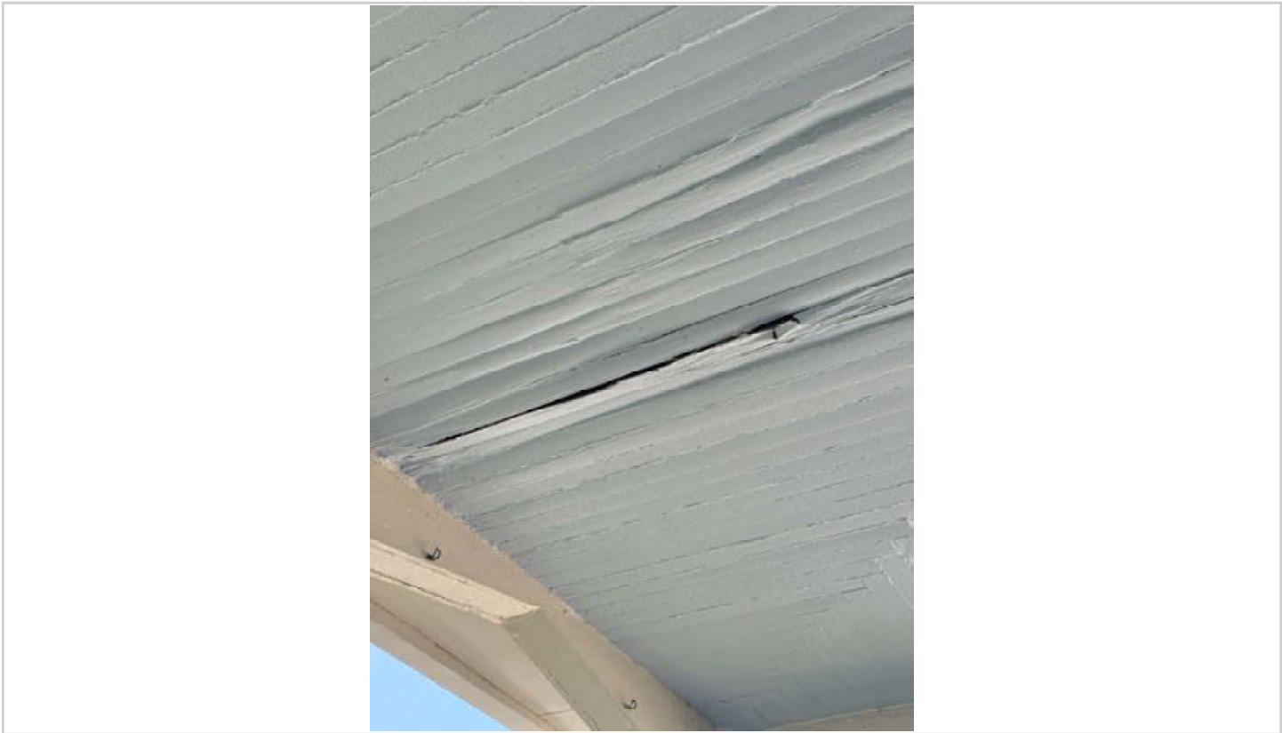
West side - Porch ceiling - Decay from roof leak
