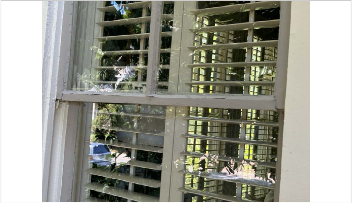
Northeast side - Window trim rot
