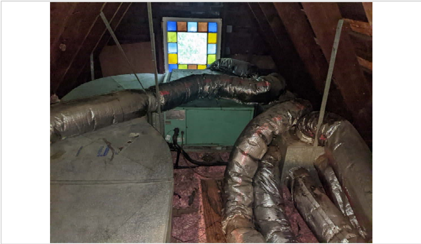
Existing air handler and duct work in the attic (west) to be replaced and modified to accommodate new heat pump. (8/9/2024)
