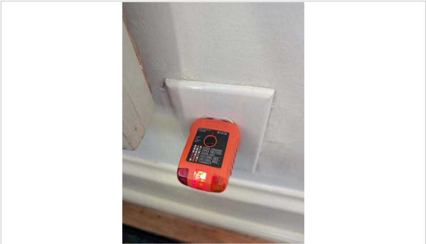
Example of an ungrounded receptacle which will be corrected to achieve proper ground. (8/25/2024)
