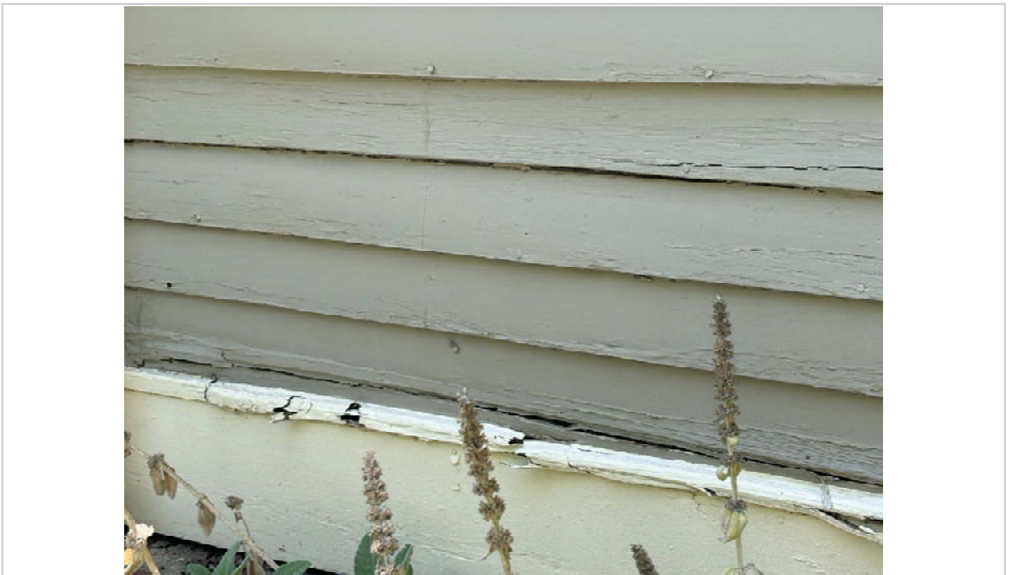
East side - Siding/Trim rot
