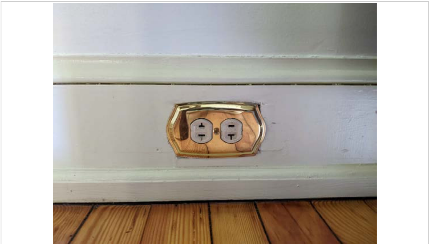
Example of a two-prong receptacle in the home to be replaced with three prong receptacles, with proper grounds added. (8/25/2024)
